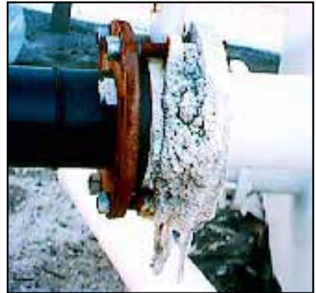
What appears to be corroding metal on Nulex tanks, is really only fertilizer crystals.
